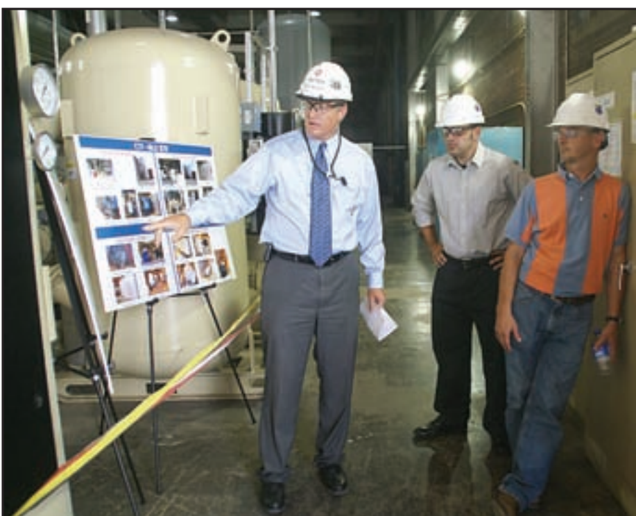
AEDC will save money thanks to a new compressed air system that will be completed at the end of 2011. The system already is saving money in maintenance and energy costs. The old system was inefficient in its use of electricity to drive huge compressor motors and the need to "bleed off" a great deal of compressed air that it didn't use.
