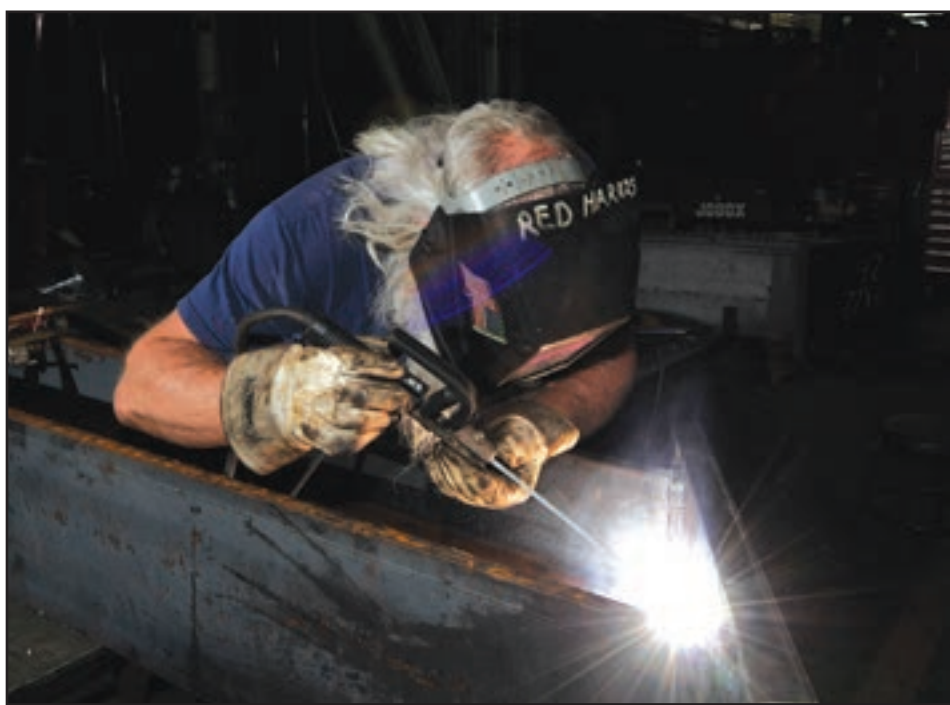
James "Red" Harris, an ATA ironworker, welds a connection of the 4T CTS Checkout Stand. (Photo by Rick Goodfriend)
