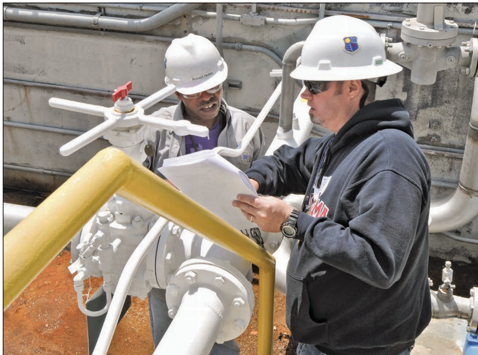
Robert Holley (left), from the AEDC Fuel Farm, and Carl McGee, with the AEDC Aeropropulsion Systems Test Facility, discuss a work instruction and a safe plan of action prior to bringing up fuel pressure for a fuel system leak check utilizing Jet-A fuel. (Photo by Jacqueline Cowan)
