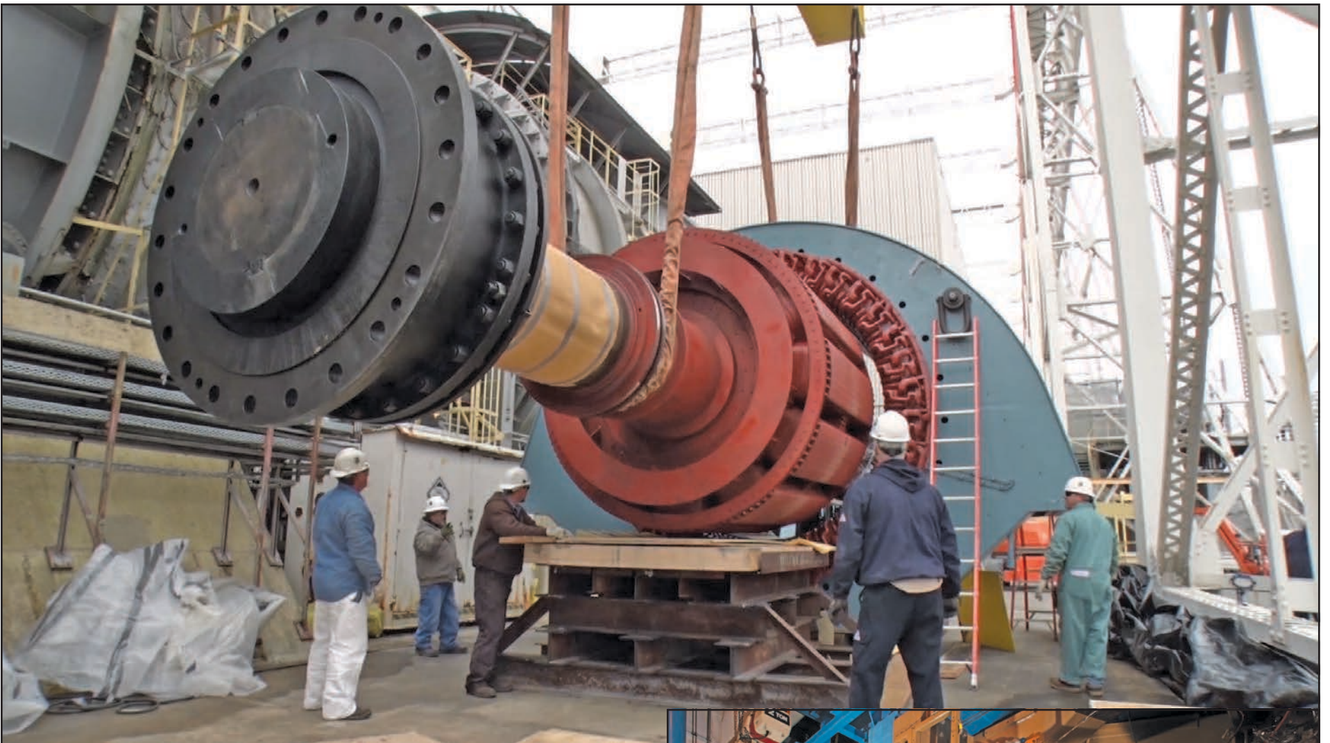
As part of an improvement project for the AEDC Propulsion Wind Tunnel, a new M4 motor stator was installed in the main drive. The function of the stator is to rotate the main compressors for the PWT 16-foot transonic and 16-foot supersonic wind tunnels. Pictured here are AEDC Propulsion Wind Tunnel craftsmen working to thread the stator. (AEDC photo)
